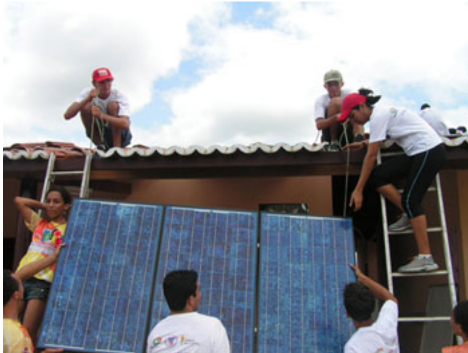
Figure 13. Youths installing solar panels to power a rural computer center, São João, Brazil
